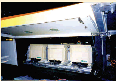
Zinc-Air Fuel Cells installed on bus
